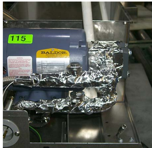
Heater strip installed [115V PF50 (Return/Suction)].
