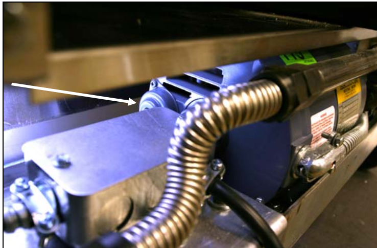
Filter Pump Reset Switch (Arrow)
