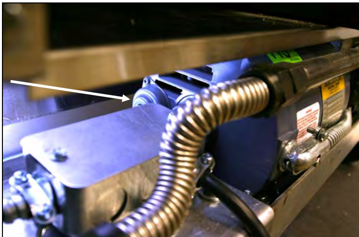
Filter Pump Reset Switch (Arrow)
